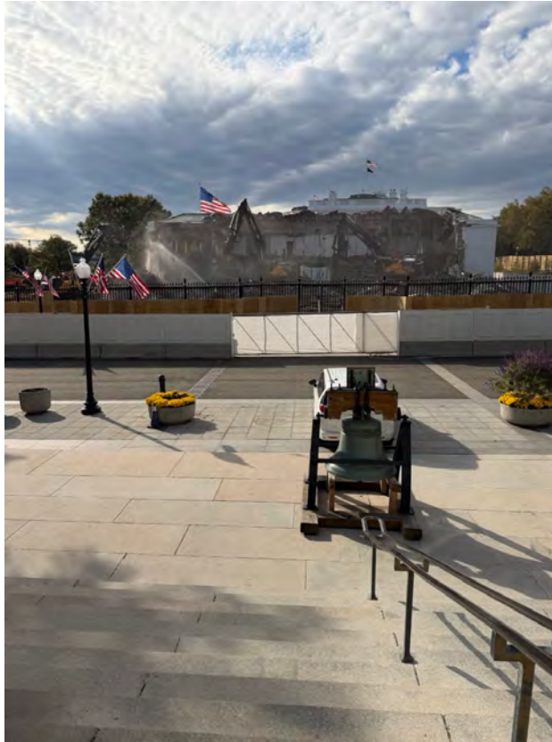
Figure 3 – View from Pennsylvania Avenue of active demolition of the East Wing, with excavators tearing into the structure behind security fencing, water spray controlling dust, and American flags lining the foreground walkway. The Washington Post.
